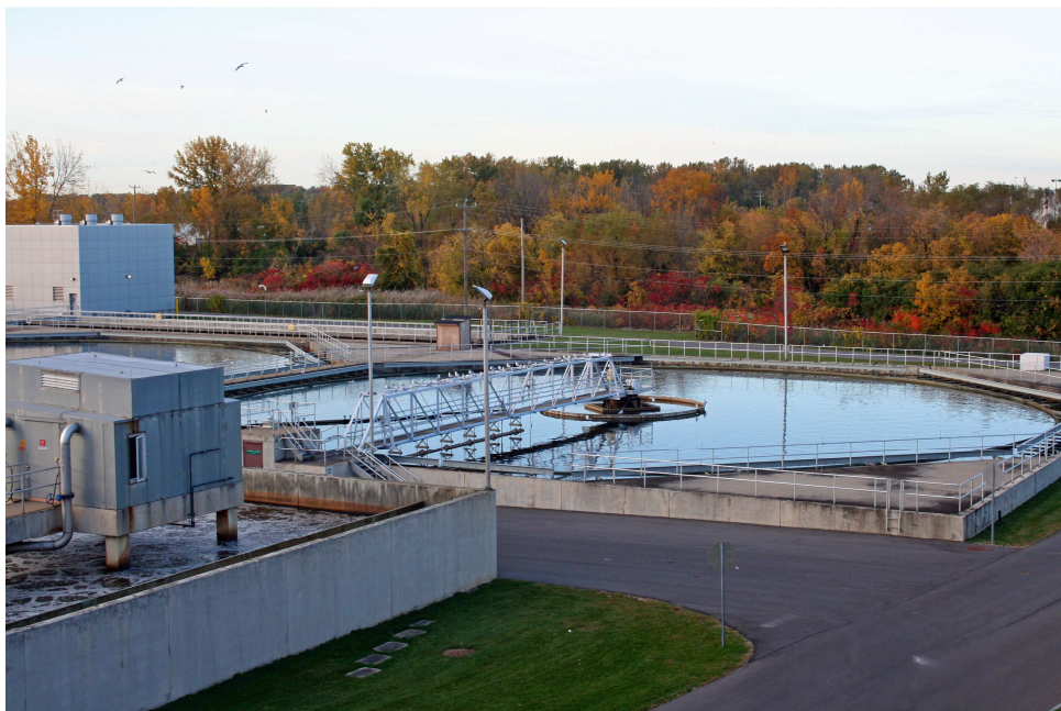
(Metropolitan Waste Water Treatment Facility)
